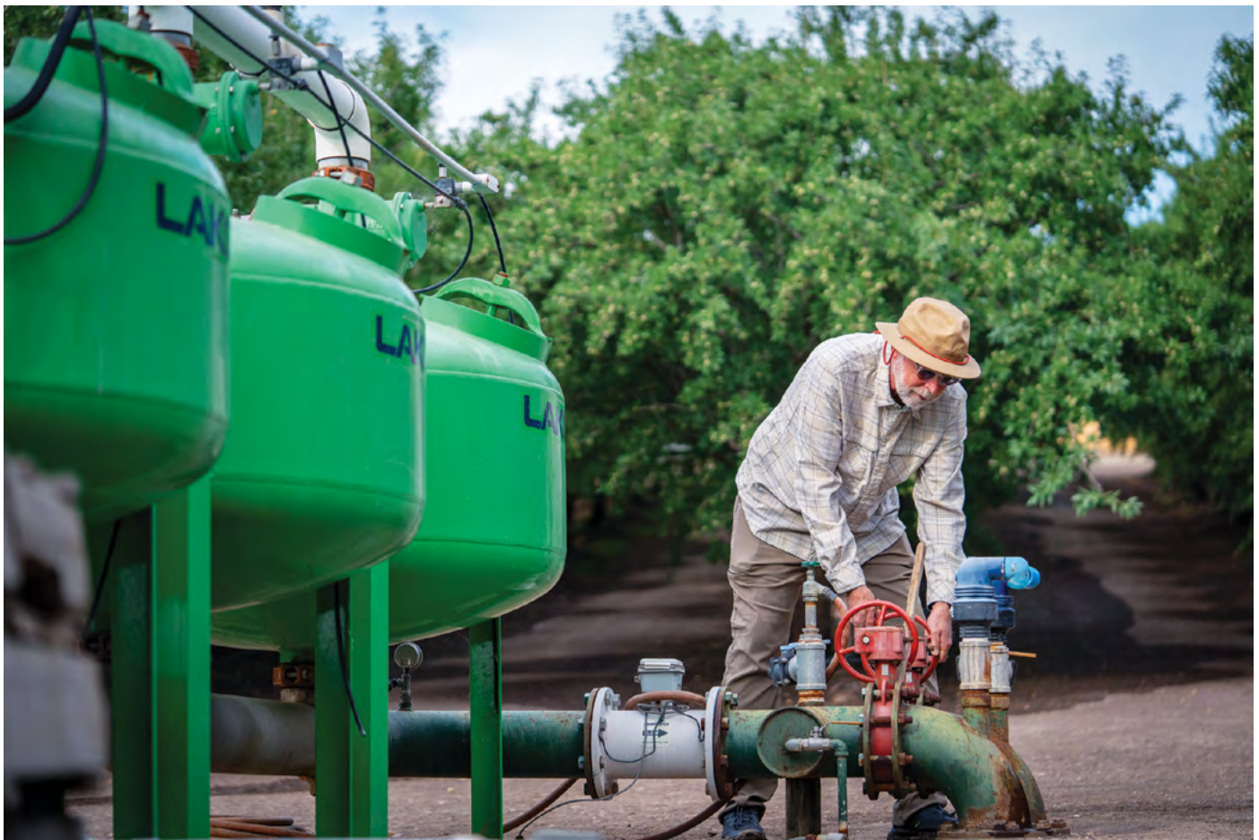
ABC's irrigation & technology adviser, Tom Devol at an irrigation pump
